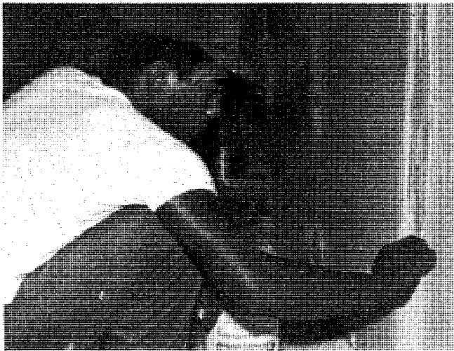
Sp4 Curtis J. Cook puts an extra effort in finishing a new wall in Delta Company, 197th Support Battalion's dayroom.
